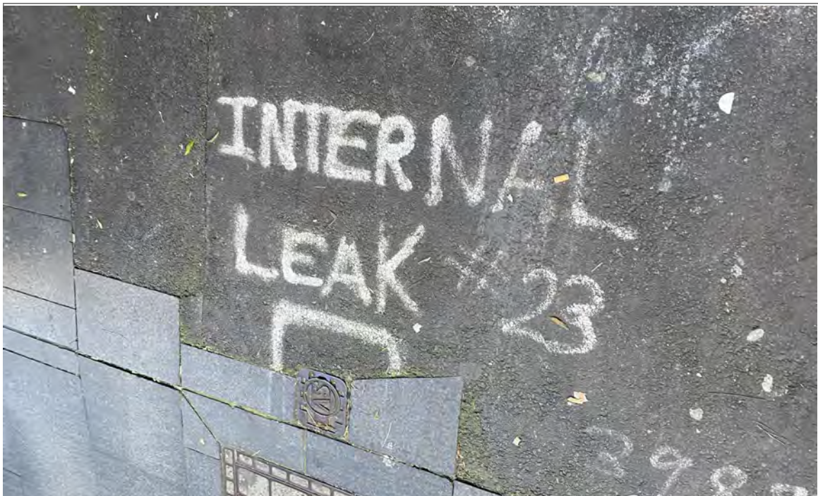
Photo 4: Internal leak marked on the pedestrian foot path along Pitt Street
